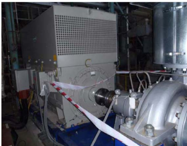
Picture 1: Pump unit
